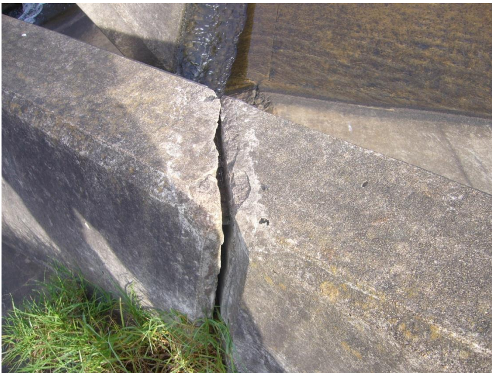
Figure 4: Baynesfield Dam: Spalled concrete on spillway due to movement of concrete structure on embankment.
