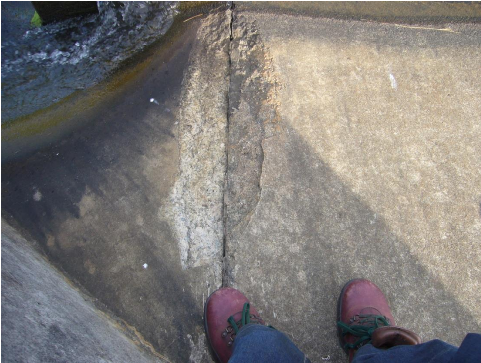
Figure 3: Baynesfield Dam: Spalled concrete on slipway due to movement
